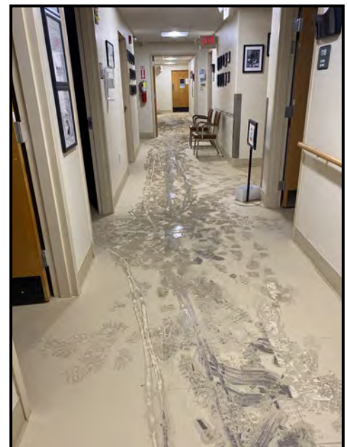
Inside the June Buchanan Clinic following the flooding.
